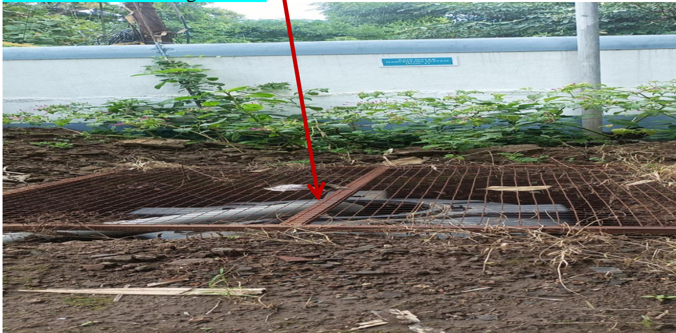
Rain water Harvesting -Unit-2
