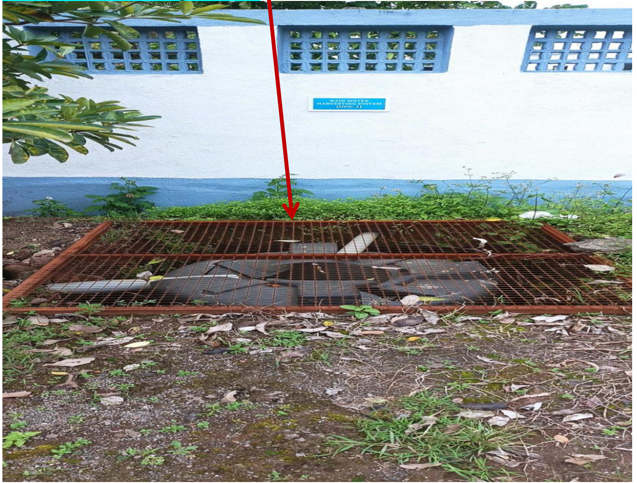
Rain water Harvesting -Unit-1
